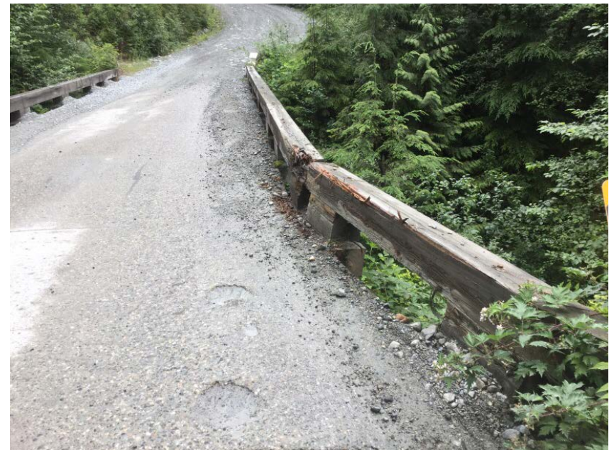
Guardrail damage downstream right bank - still functional
