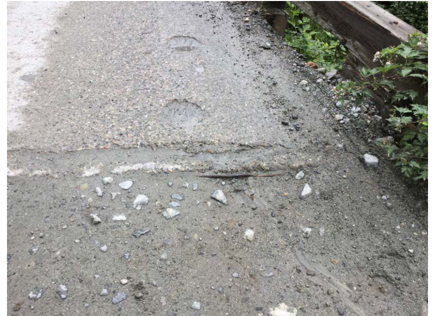
Exposed rebar on right bank ballast wall
